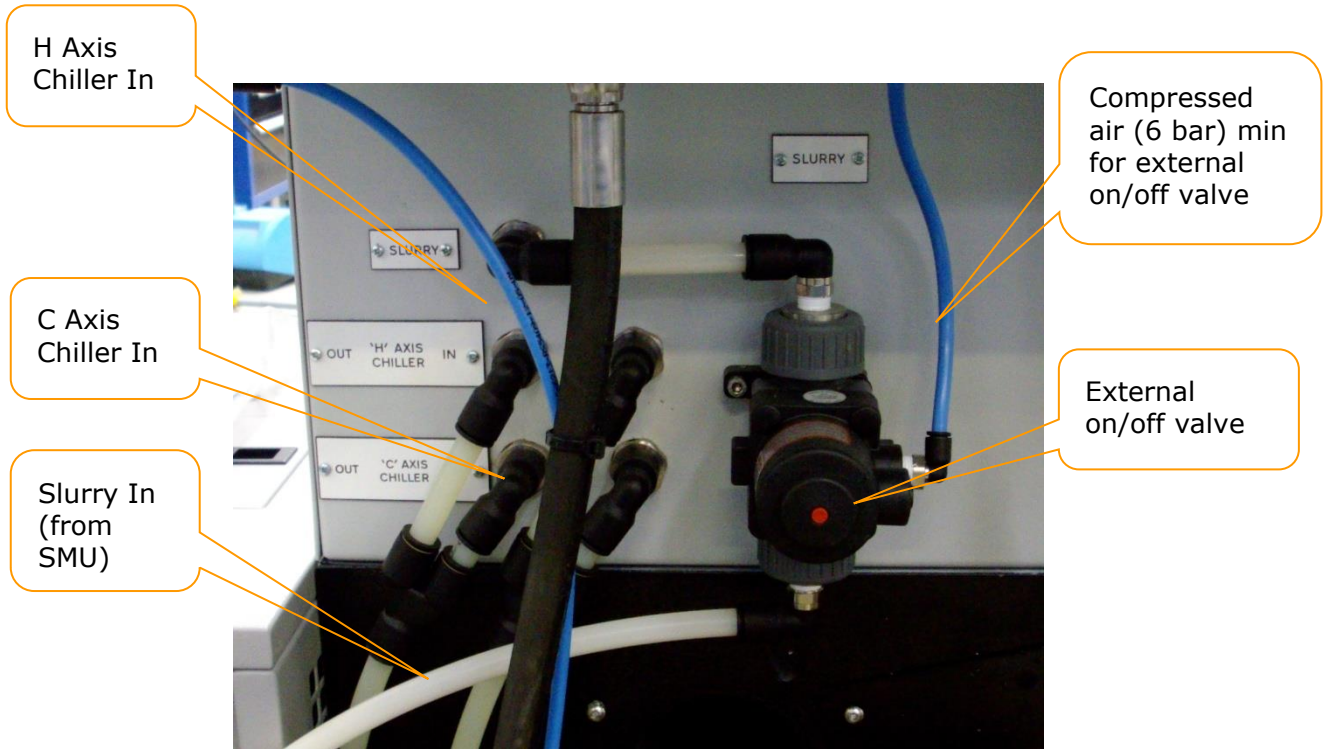
Figure 8: Supply connections to IRP600 machine
